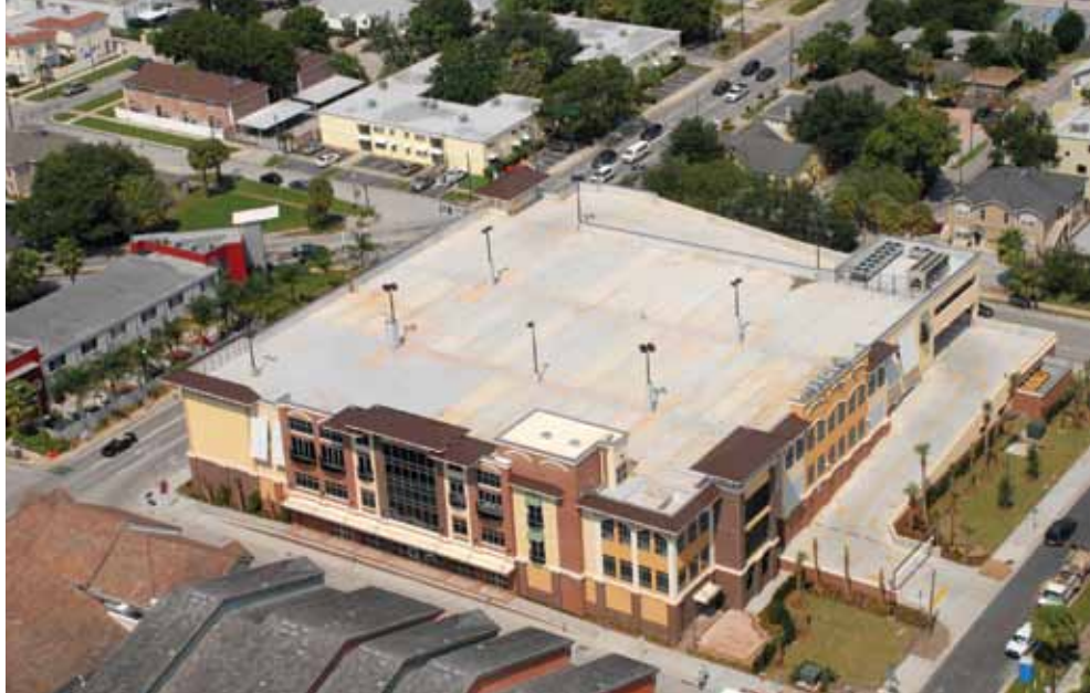
The tight site required the structure to be built from the inside out, positioning the crane inside the footprint and working across the building before backing up to erect the next set of bays. When the crane finished the final portion, the speed ramp to the parking levels was built as the final piece.
